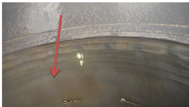
Figure 10: Photo of liner number 1 after 10319 running hours – machining marks visible in the top
