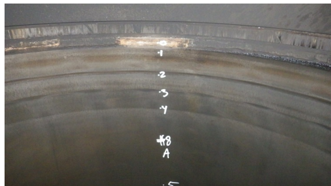
Figure 12: Photo of liner number 8 after 4600 running hours – machining marks not visible
