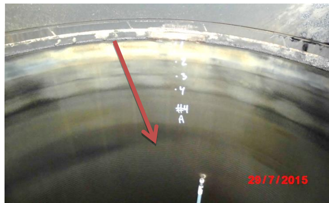
Figure 11: Photo of liner number 4 after 9260 running hours – machining marks visible 300mm from the top
